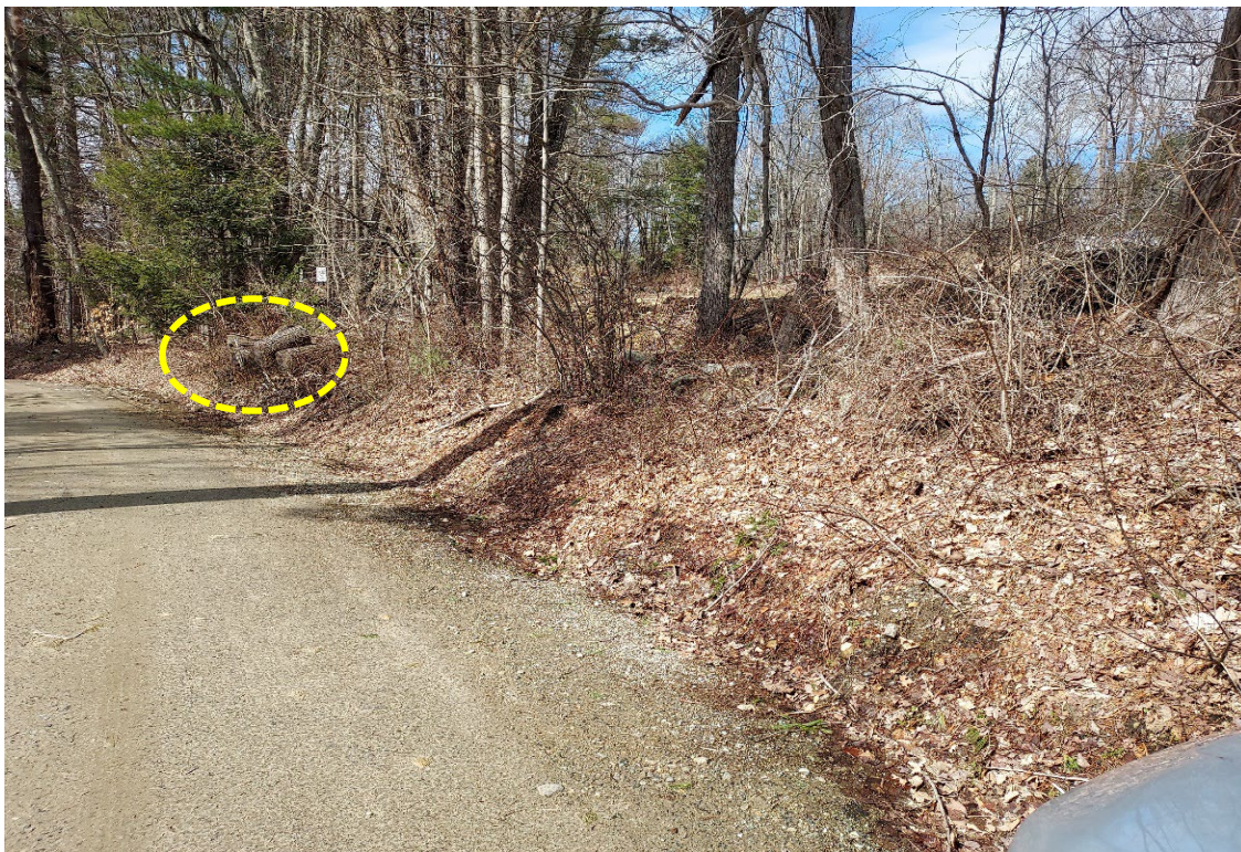
Photo 2 – Looking westerly along Lake View Drive. The pond is atop the embankment in the right of the photo. The circled area points out the location of the sole outlet pipe and the seepage area noted in the following photo.
