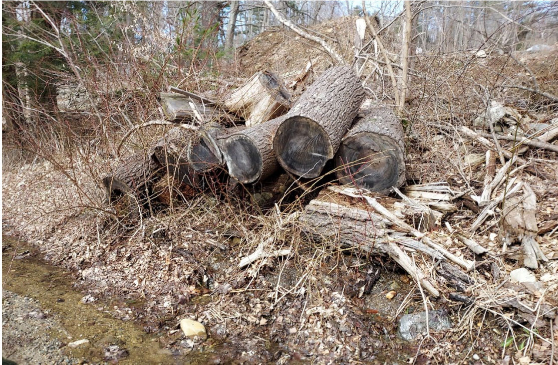
Photo 3 – The outlet seepage area pointed out in the previous photo. The seepage extends over an approximate 6-foot width emanating from under the pile of logs.
