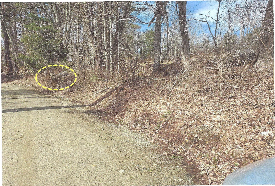
Photo 2 – Looking westerly along Lake View Drive. The pond is atop the embankment in the right of the photo. The circled area points out the location of the sole outlet pipe and the seepage area noted in the following photo.
