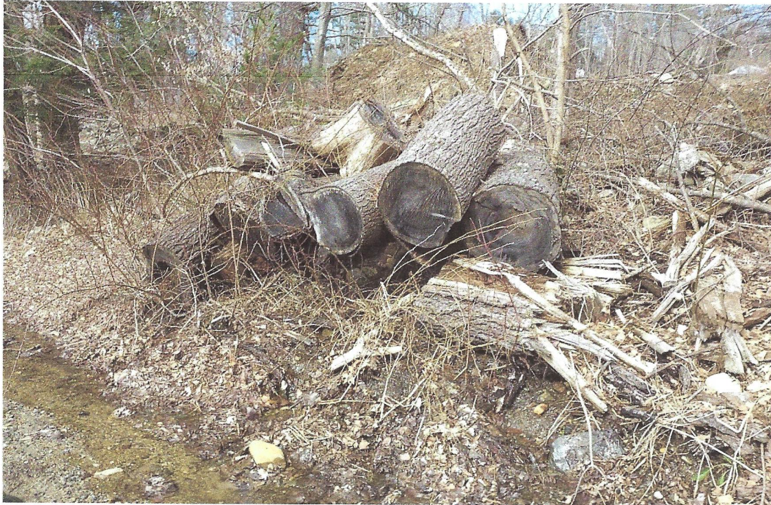
Photo 3 – The outlet seepage area pointed out in the previous photo. The seepage extends over an approximate 6-foot width emanating from under the pile of logs.
